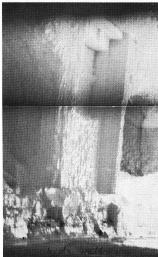
Figure 11. Collapsed AZS wall between both burners.
