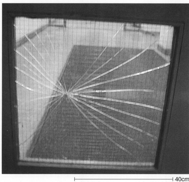
Figure 1. Typical damage to a wired glass window caused by a foreign body impact of low energy.
